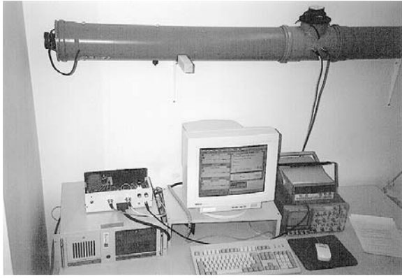
Figure 3: The complete ANC demonstration system consists of a duct, a PC-rack equipped with a DSP and a data acquisition board, and an audio box including microphone and power amplifiers.
